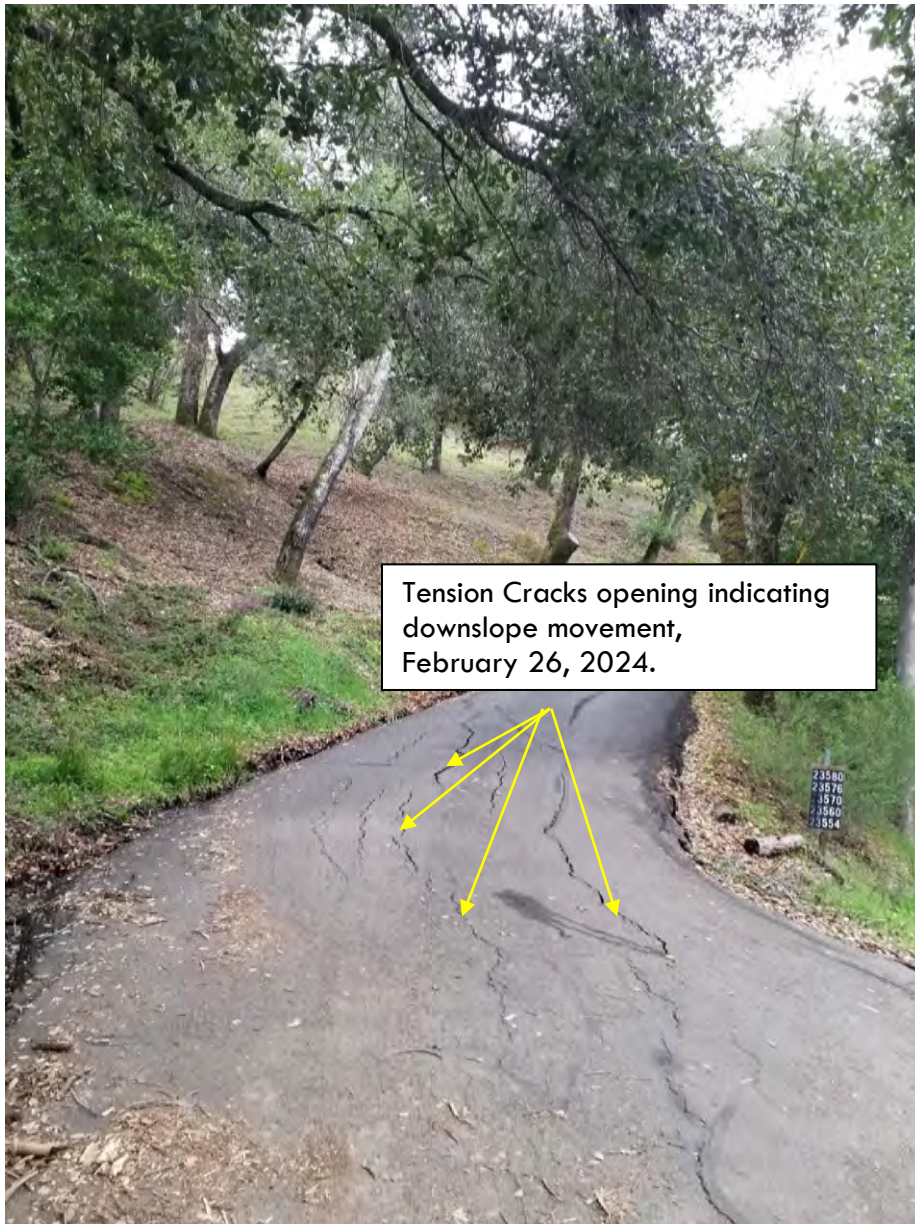
Exhibit 7 February 26, 2024, Tension Cracks
