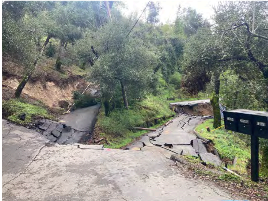
Exhibit 2 Scarp and Damage on Mountain Charlie Road, Looking South at PM 1.63
