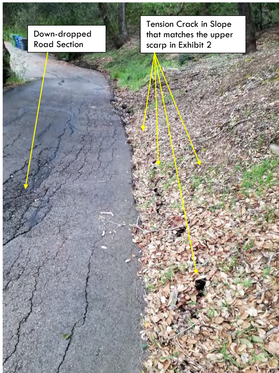
Exhibit 8 Tension cracks, down-dropped road, tension crack in slope, February 26, 2024
