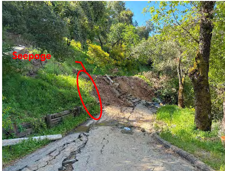
Exhibit 4 PM 1.63 Looking South, Seepage Area Shown Above Road
