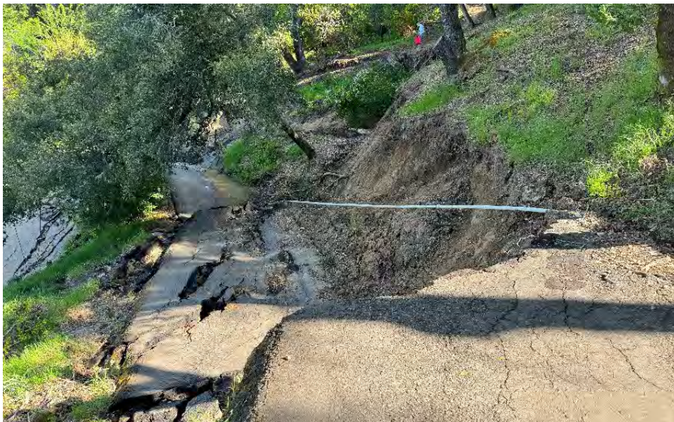
Exhibit 3 Scarp on Driveway, Looking North at PM 1.63
